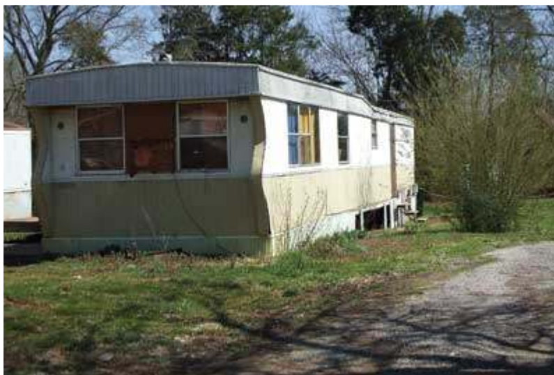
(2) This older mobile home shows the effects of age and neglect. Openings in the walls and exterior covering can allow
