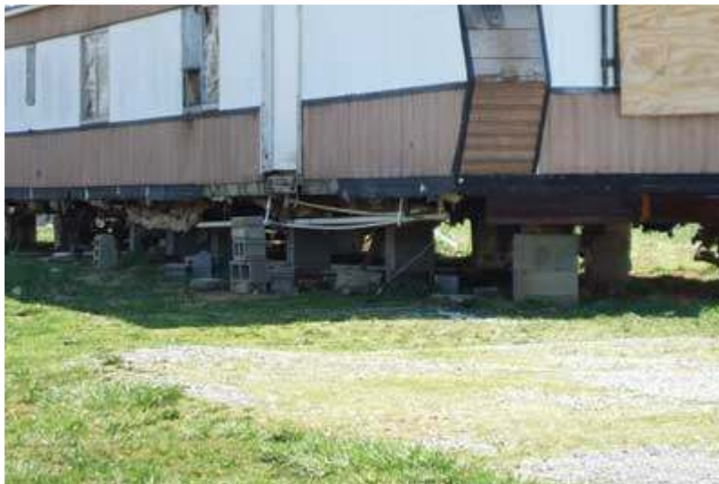
(8) Pipes, wires, insulation, tie-downs, cinderblocks, tires, and axle assemblies can all be found under most mobile homes. These items are dangerous when attempting to rescue a firefighter.
